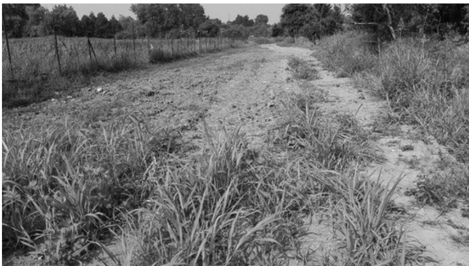
Figura 10 – Vista D post operam
